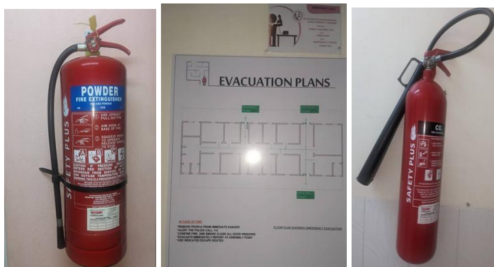
Figure 17: Firefighting materials and fire indication signals
