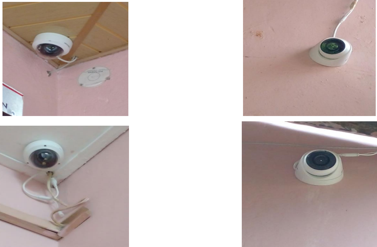
Figure 16: CCTV Cameras for internal security
